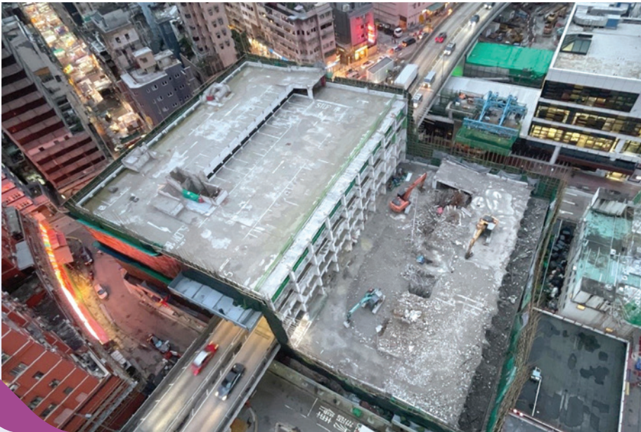
Part of Yau Ma Tei Carpark Building demolished was only one wall away from the Gascoigne Road Flyover.
