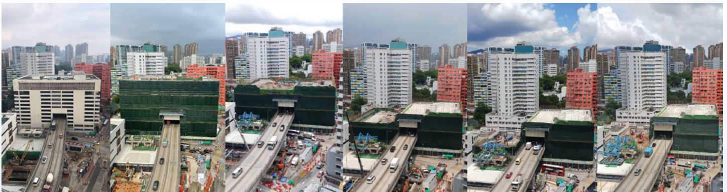
Time-lapse images, from April to August 2021, showed progress of the first phase of Yau Ma Tei Carpark Building demolition works.
