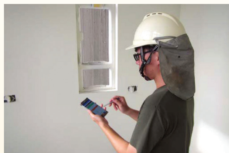
DCSMS enables site staff to conduct site supervision more effectively with smartphones.
