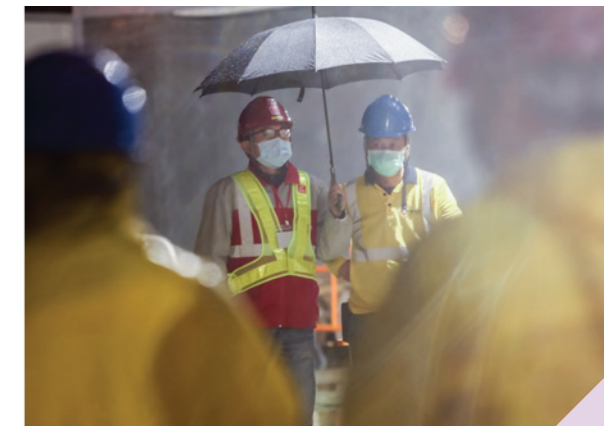
Frontline workers performed diligently and rigorously irrespective of the harsh working environment, coldness and rain, for accomplishment of the construction work.
