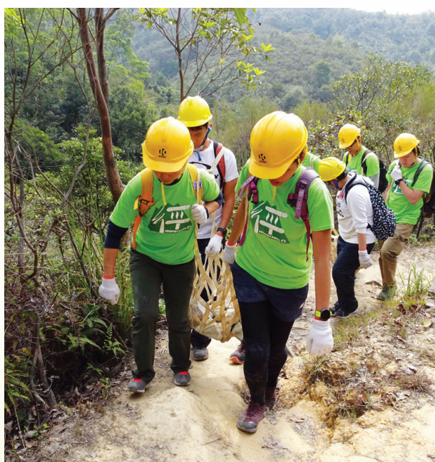
Trail volunteers work together to carry the construction materials for trail works.
